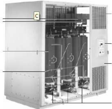
Cast Coil Substation Transformer
